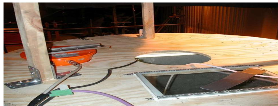
Top of silo with MGD detection system
