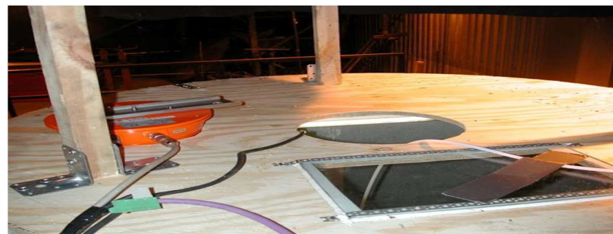
Top of silo with MGD detection system
